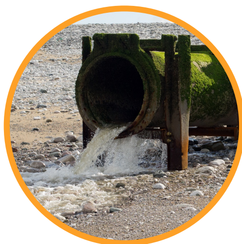
An overflow pipe on the beach Credit: MCS/Kate Wilson
